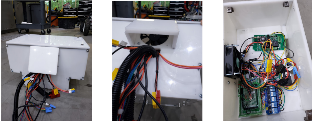
Figure 3: New Electrical Enclosure
