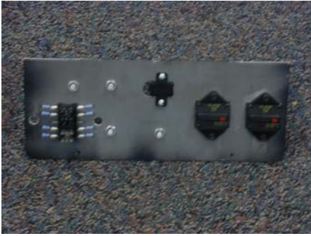
Figure 8: MARC Circuit Breaker Panel
